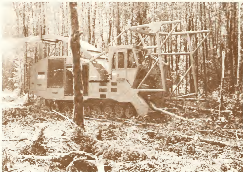
This machine prepares an 8-foot-wide, 1-mile-long strip for replanting while converting debris into usable chips as it moves along.
